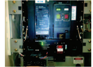
Remote Racking System
