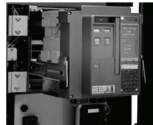
Deadfront, Drawout Breaker
